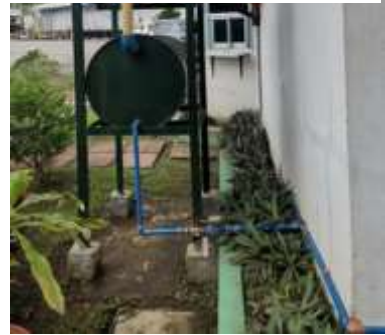
Tacloban Terminal's rainwater harvesting set-up
