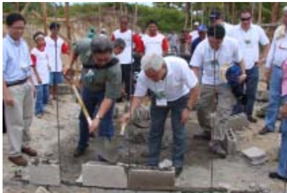
Building a community, rebuilding hope. Petron Chairman Nicasio Alcantara (3rd from left, foreground) leads partners in constructing the Tulong Kapwa-GK Energy Village with (from left) Department of Energy Secretary Raphael Lotilla, National Transmission Corporation President & CEO Dr. Alan Ortiz, Mirant Philippines Foundation Executive Director Roberto Calingo, Gawad Kalinga Executive Director Antonio Meloto and Southern Leyte Governor Rosette Lerias (partly hidden)
